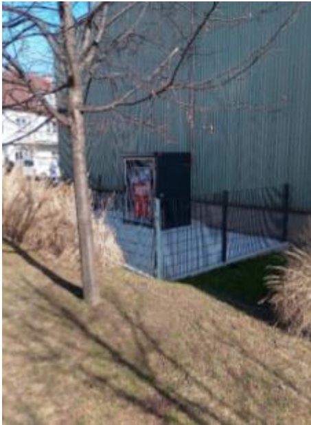
Safety storage of the hydrogen supply in a gas cylinder storage outside the technical center of the Chair of Thermal Processing Technology (MUL)
